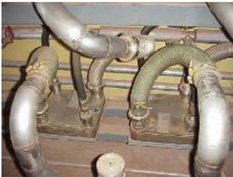
The two B60s installed at IRCA, covered with cocoa dust.
